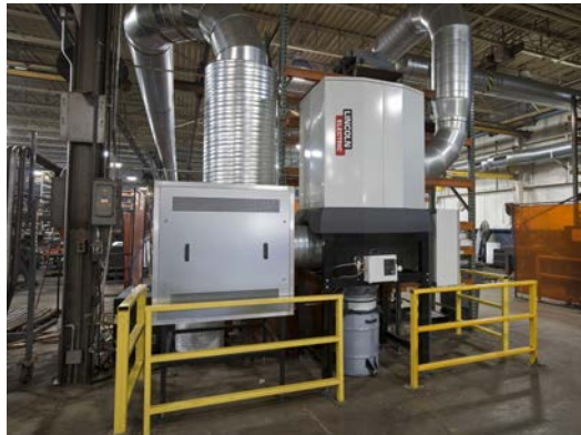
Push/Pull System installed at Elgin Sweeper Company
